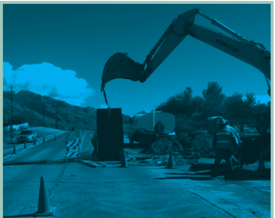
Construction on the Magee Road, Shannon Road to La Canada is nearing completion. With the mainline now complete construction crews are making the final tie-ins along side streets.
